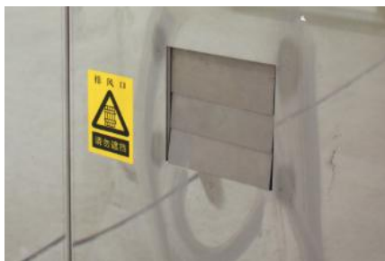
Exhaust hot air outlet
